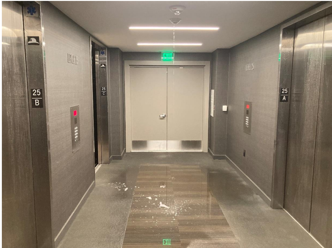
Figure 5 – Image of flooded elevator area
