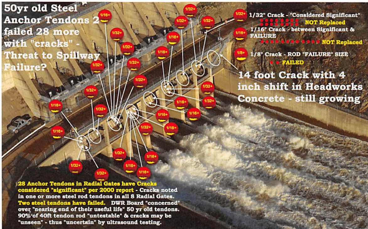
Figure 1: Broken (2) and cracked (28) spillway gate control anchor tendons.
